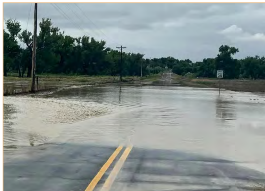
Figure 89:Flooded Road in Pueblo County.
